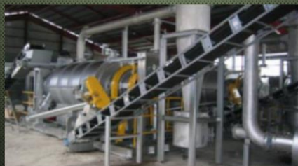
K2 CARBONIZATION PLANT ROTARY KILN SEMI-AUTOMATED
